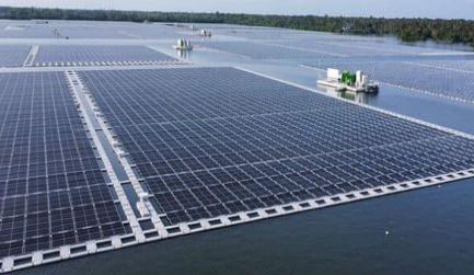
Ramagundam Floating Solar PV Project
